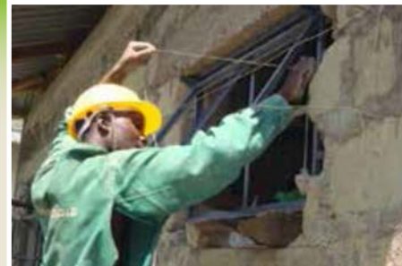
Construction worker ensure precision of standards are adhered to at Tamu Law Court.
