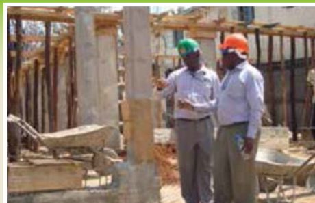
Construction engineer and Clerk of Works from DBS ensure quality materials are used at Oyugis court construction.
